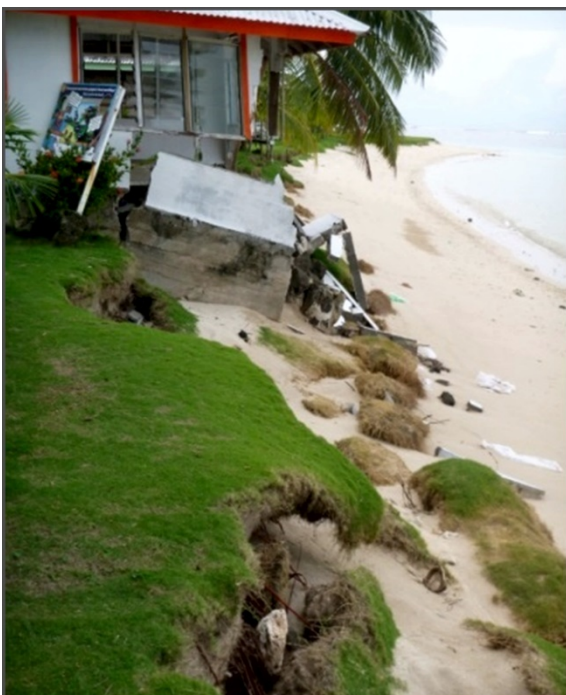
Figure 16 Erosion, Cyclone Gita, Lelepa Village Savai'i
